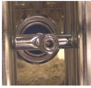
No water valve in place
